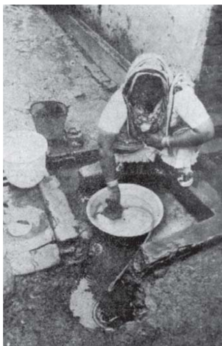
Broken watertap, faucet below sewage water level, situated next to latrine and gutter. Dinking water is obtained through a hose connected to the faucet.
